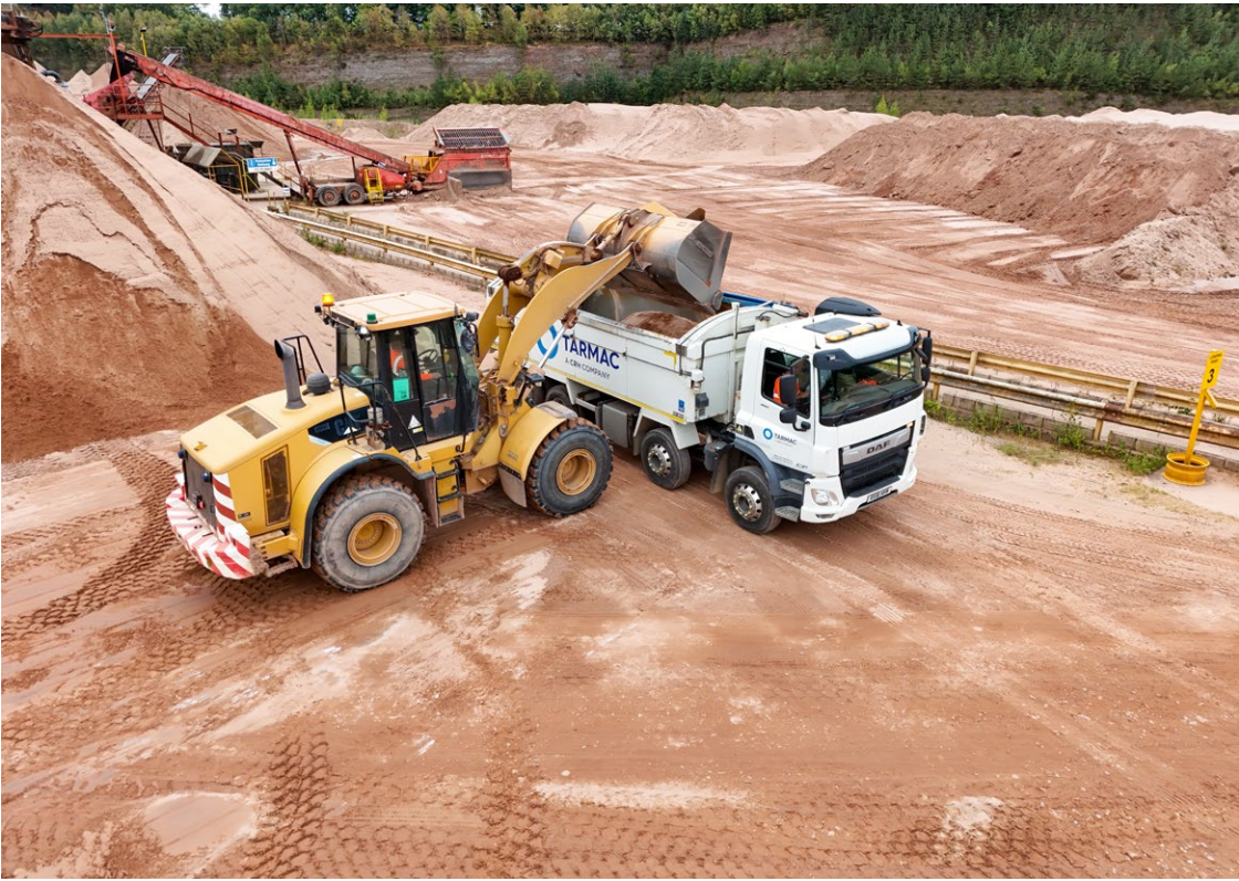
A loading cab loading materials into a tipper ahead of delivery offsite
