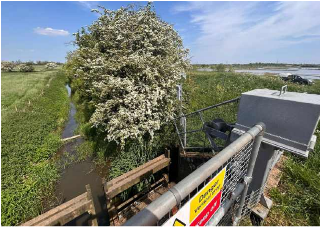
CCTV has been installed on Slough Dyke for early response to flooding incidents
