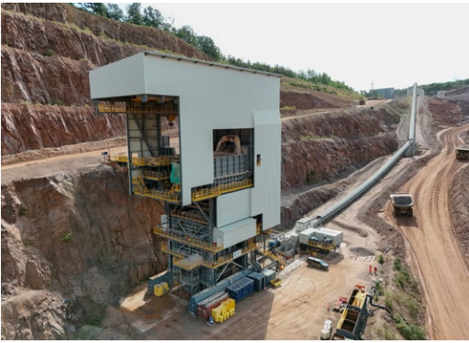
New Primary crusher
