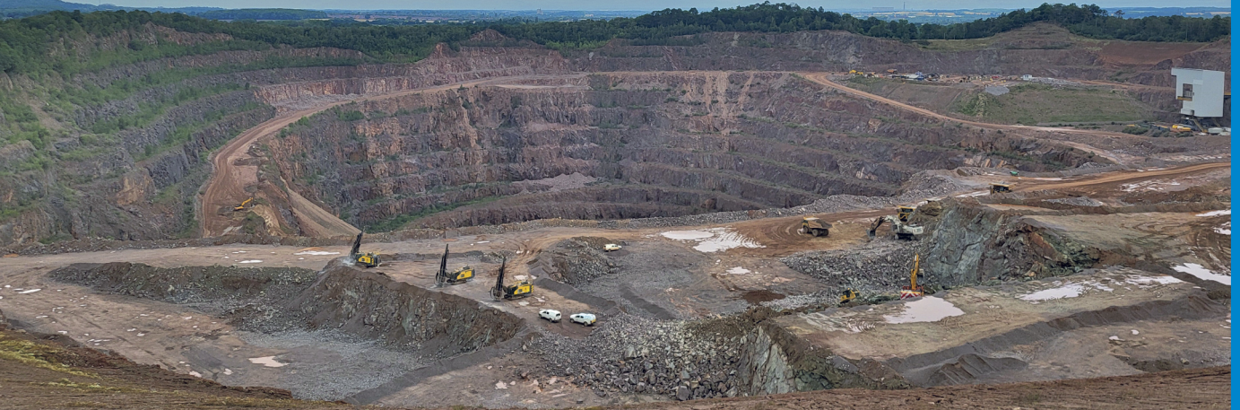
Utilising specialised machinery, numerous holes are drilled in a defined pattern which are then loaded with high explosives and detonated using sophisticated electronics for precise timing to maximise rock breakage and control direction.
