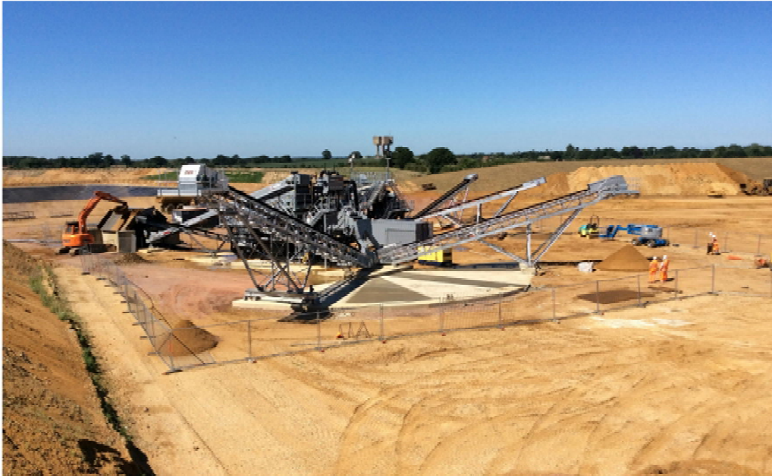
The processing plant at Stanninghall Quarry
